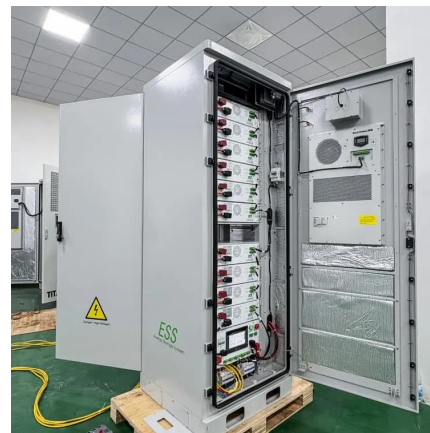
Off grid container power systems -- Off-Grid Installer
