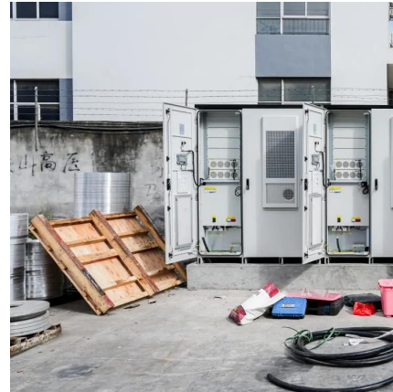
Energy storage container, BESS container
