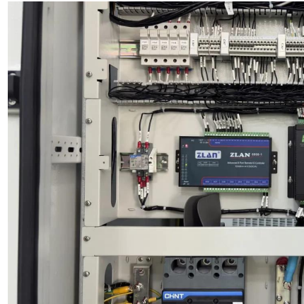
Honiara energy storage cabinet
