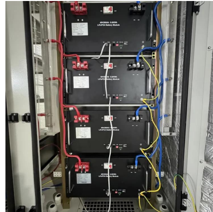
Energy storage container, BESS container
